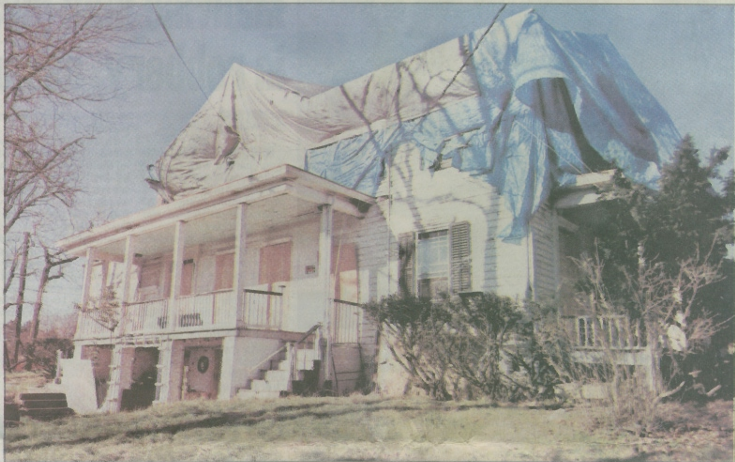
Tarps and plywood cover the windows and roof of the Metlar-Bodine House Museum on Friday after an electrical fire devastated the house in July. Officials hope to have a temporary roof on the house by next month, with a permanent one when there is enough money.
